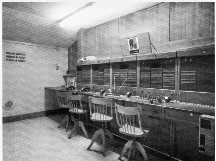
Telephone Exchange at Fort Scex
